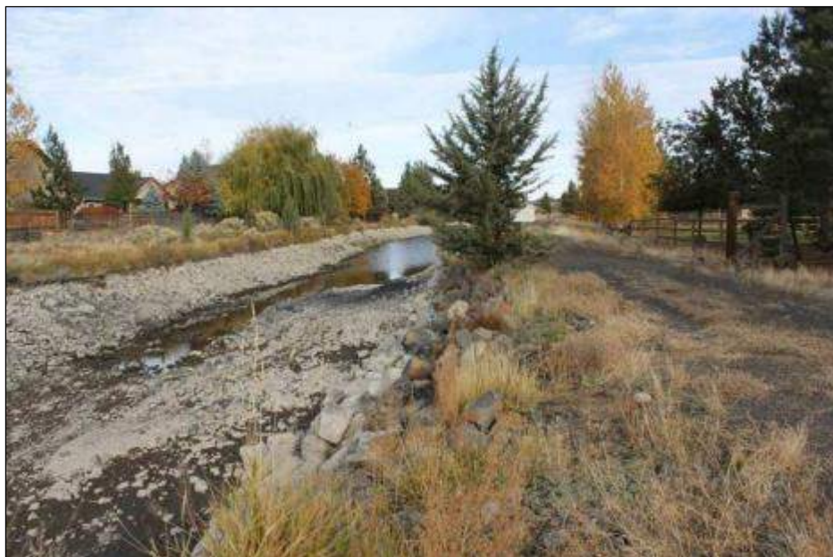
Segment 1: City of Bend on left of canal centerline. At-grade cut on left (west) side of canal; embankment on right (east). Rural county livestock farms on right. Photographer looking north.
