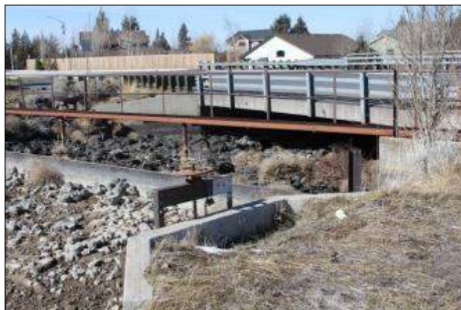
Photo shows some of the alterations to the canal in Stretch 4, immediately south of historic district: the new gate to a piped A-4 Lateral, a low head check, and a bridge at Empire Avenue. The bed under the bridge has been paved to prevent erosion. Photographer looking northwest.
