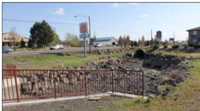
Canal leaves a 1,100' segment of pipe and enters a culvert under Odem Medo Road in Redmond. Highway 97 is in background. Photographer looking south.
