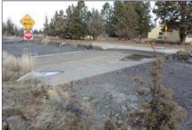
SEGMENT 5: 55' wide by 46' long concrete flow-measuring weir constructed in the canal bed in 2012. Photographer looking northeast.
