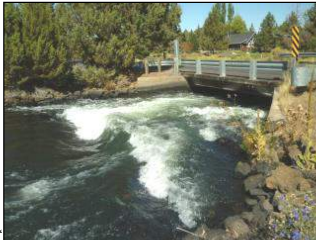
SEGMENT 2: Water leaves an 81-foot wide, rocky area and rushes under the 20-foot wide Old Deschutes Road Bridge. Photographer looking northeast. 37
