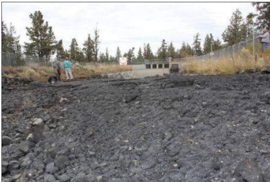
Segment 5: Men are standing on lava flow in the canal bed at the northern Historic District boundary line. The red sign is hanging on a wire at the Section line between Sections 10 and 15. The structure is outside the historic district in Section 10 and is the intake for the 2.25-mile piping project for the Juniper Ridge Hydropower project. Photographer looking north.
