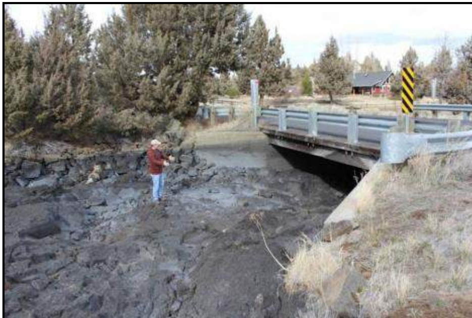
Segment 2: Old Deschutes Road Bridge. Jeff Perreault M.S. stands on lava flow. Photographer looking northeast to goat farm at red house and barn (right).
