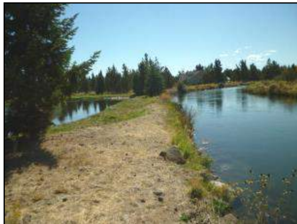
A smooth, deep area in the Pilot Butte Canal Historic District (Cooley Road – Yeoman Road Segment). The irrigation pond on the left is the altered historic Houston Pond. The embankment is about two feet tall in this area. There is no ditch rider road on the embankment. Photographer looking south. 31
