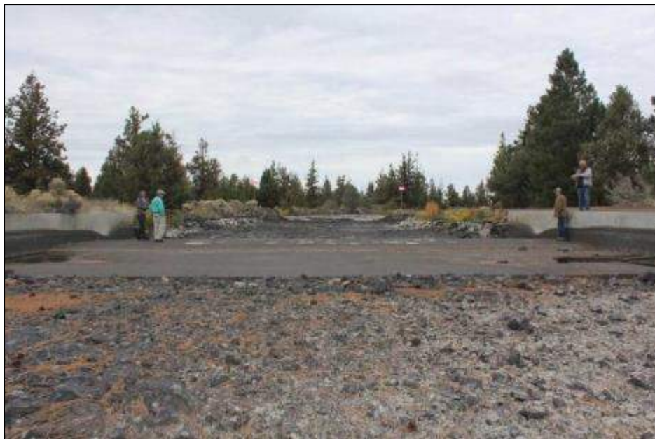
SEGMENT 5: The canal bed at its northern end is nearly flat and is wide and shallow. The surveyors are standing beside and in the 2012 concrete trapezoidal flow-measuring weir structure that was constructed in the existing canal bed. Photo looking north.
