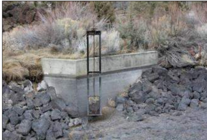
SEGMENT 2: Non-historic metal wheel control, threaded screw lift rod assembly, metal slide gate, concrete headwall and corrugated steel pipe. Photographer looking southwest.
