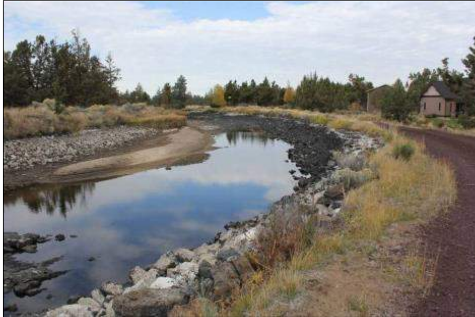
Segment 5: Red cinder covers part of the top of the embankment. This is a gently curving stretch of canal with smaller-diameter loose rock and lava flows in the canal bed. It has riprap on side slopes and standing water with silt piles. Photographer looking northeast.
