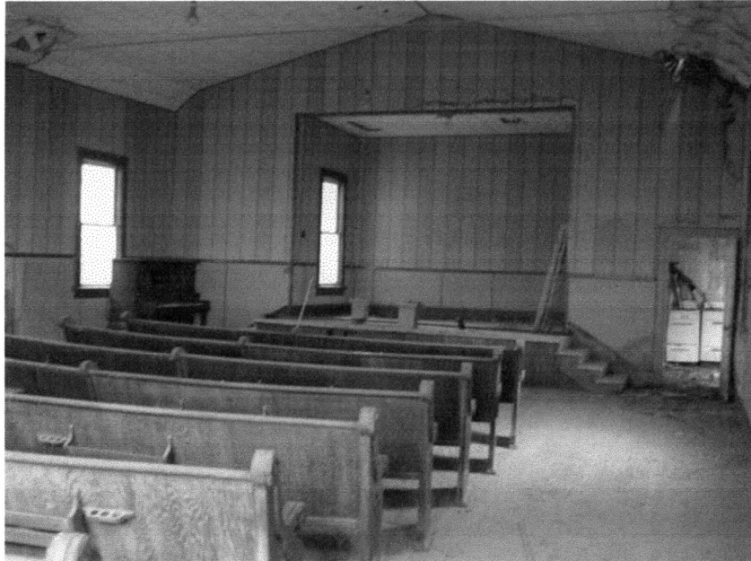
Figure 8 The raised platform floor of the north chancel extends a few feet into the main space and terminates in a slight convex curve toward the seating. The kitchen is seen through the doorway at right. Tallgrass Historians L.C.
