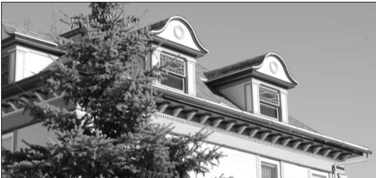
Case House, 215 2 nd St SW, dormer and cornice detail, looking northeast (Svendsen Tyler, photographer, 2014)
