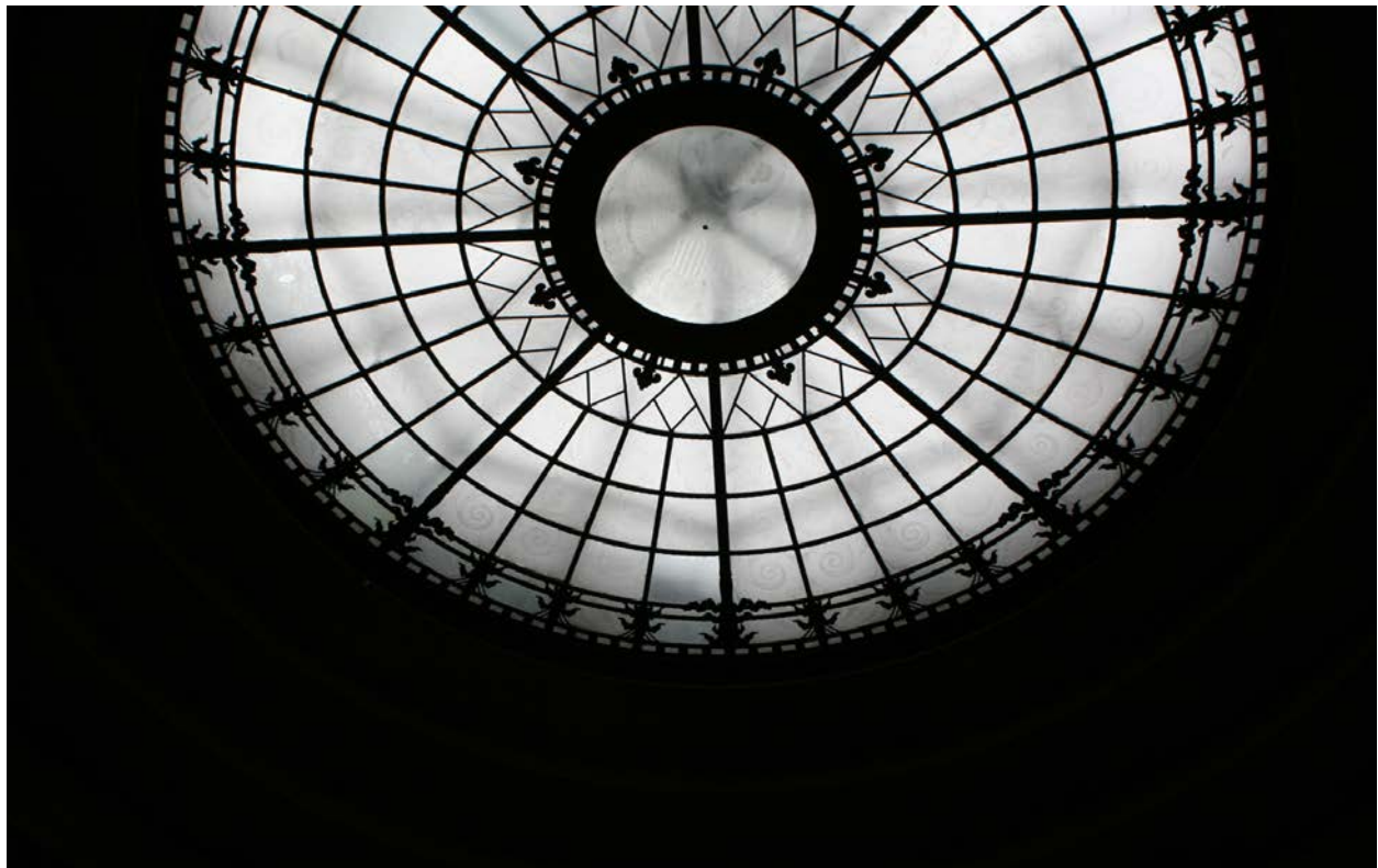
Figure 25. The large circular skylight of the Memorial Building is composed of bronze and multiple panes of etched glass, originally color-tinted. Laura L. Knott, October 19, 2011.
