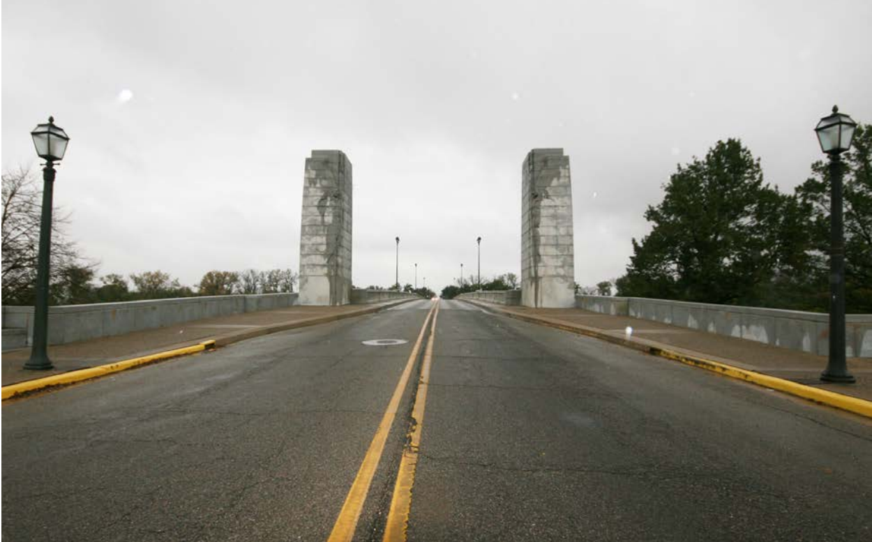
Figure 8. View looking west from the Lincoln Memorial Bridge Approach. Laura L. Knott, October 18, 2011.
