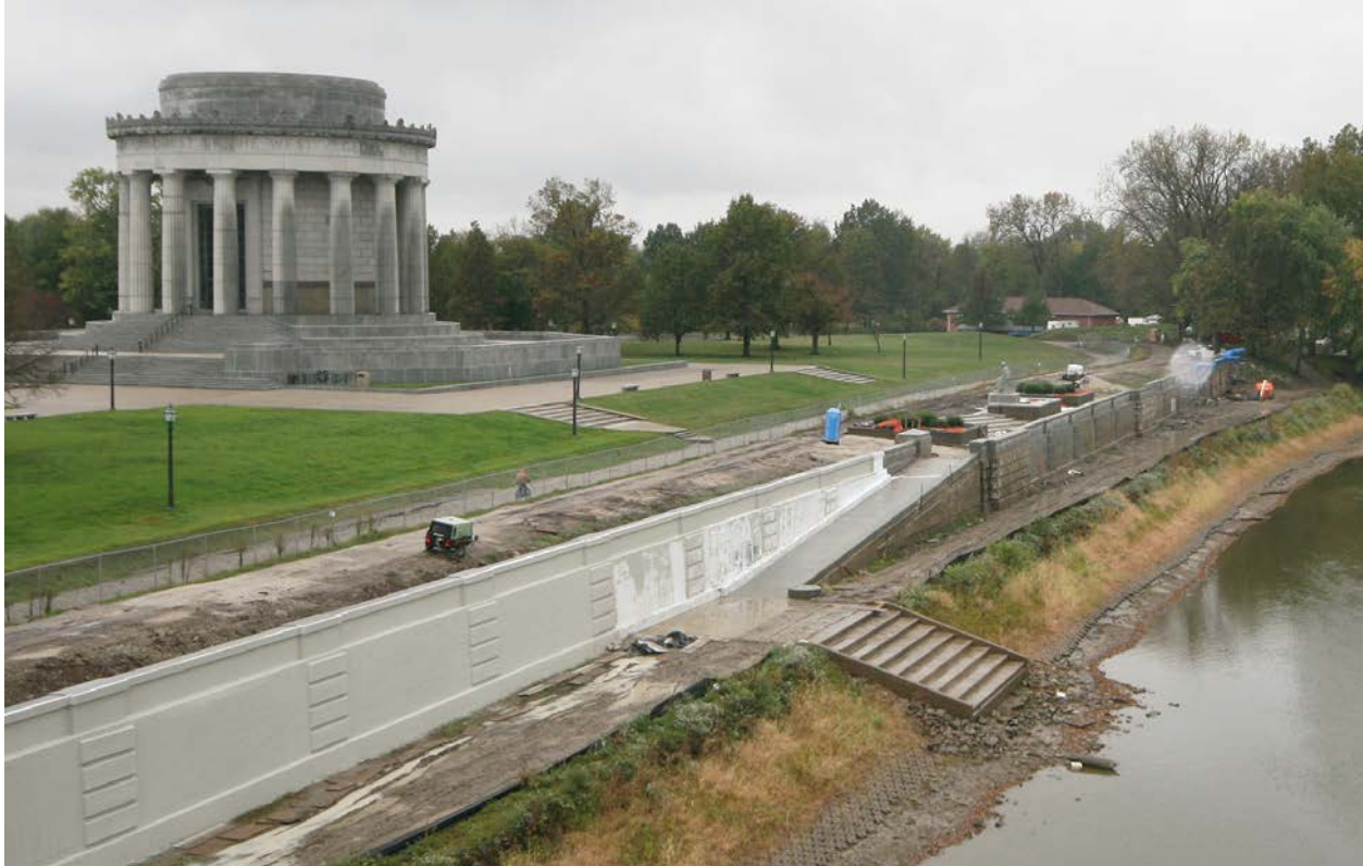
Figure 16. Vigo Plaza, river retaining wall, ramp, and stairways under renovation. Laura L. Knott, October 18, 2011.
