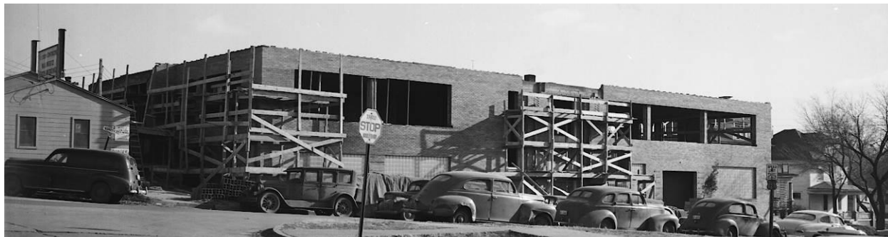
Figure 3: View of the Central Annex's north and west facades during construction (Courtesy of Sioux City Public Museum)
