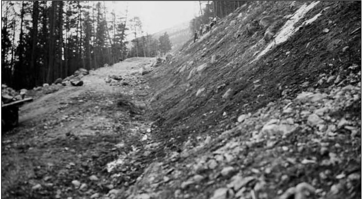
Figure 28. Construction of a new curve of Fall River Road below Horseshoe Park. (source: Superintendent's Monthly Report April 1934 [Rogers 1934a]).
