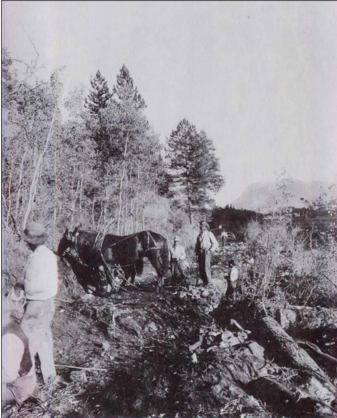
Figure 25. Constructing Fall River Road, c. 1915 (source: W. T. Parke Collection, Rocky Mountain National Park. Reprinted from Fall River Road Historic American Engineering Record CO-73 [Quin 1993a]).
