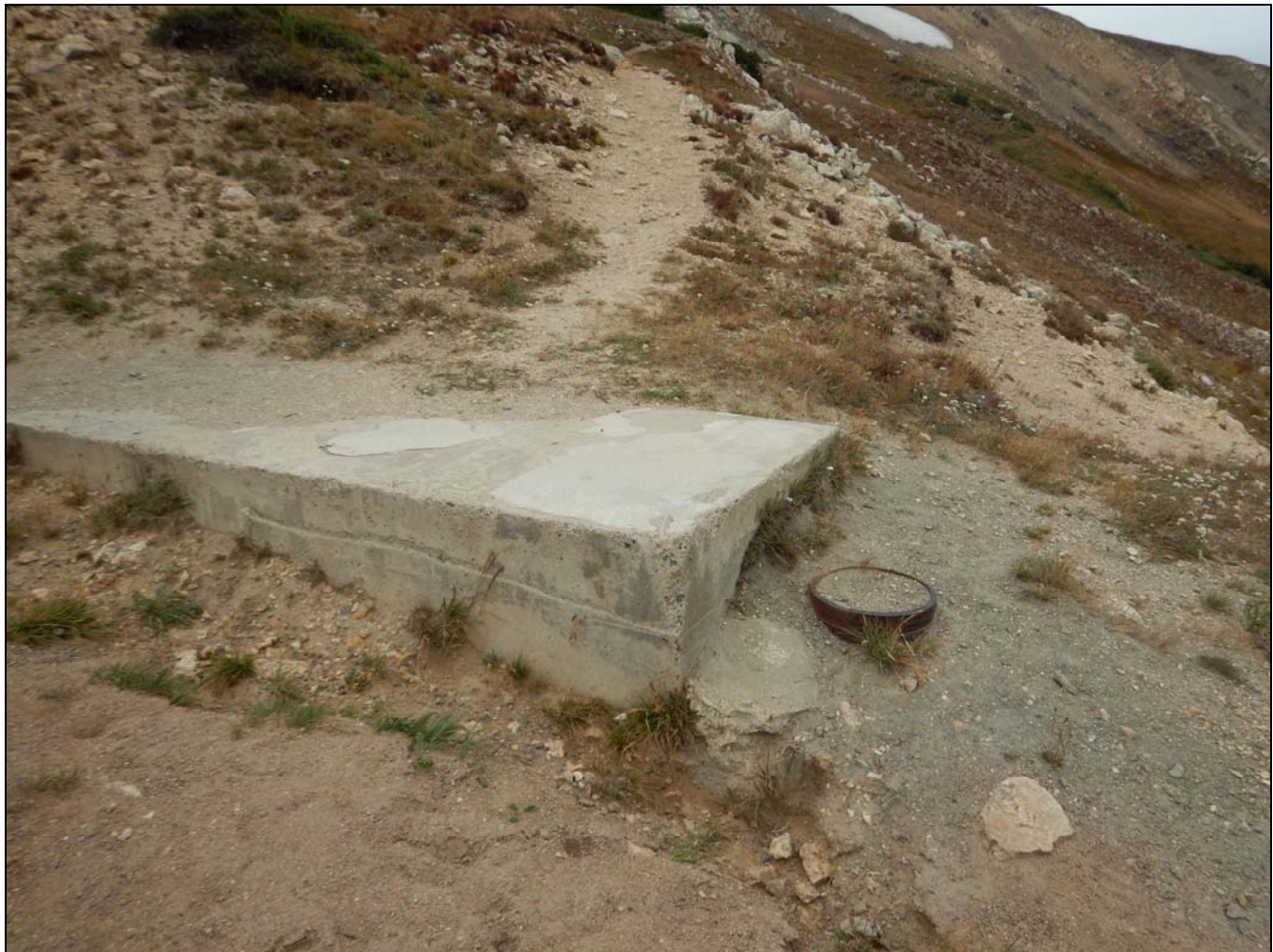
Photograph 12. Concrete pad/wellhead, camera facing west. CO_LarimerCounty_Fall River Road_Amendment_Boundary Increase_Rocky Mountain National Park MRA_0012
