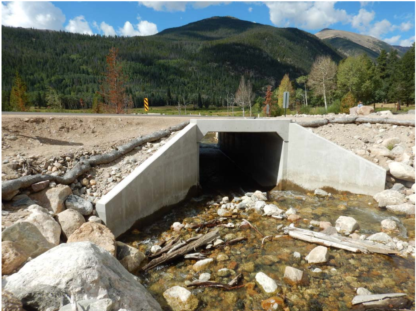
Photograph 2. Concrete box culvert, camera facing east. CO_LarimerCounty_Fall River Road_Amendment_Boundary Increase_Rocky Mountain National Park MRA_0002
