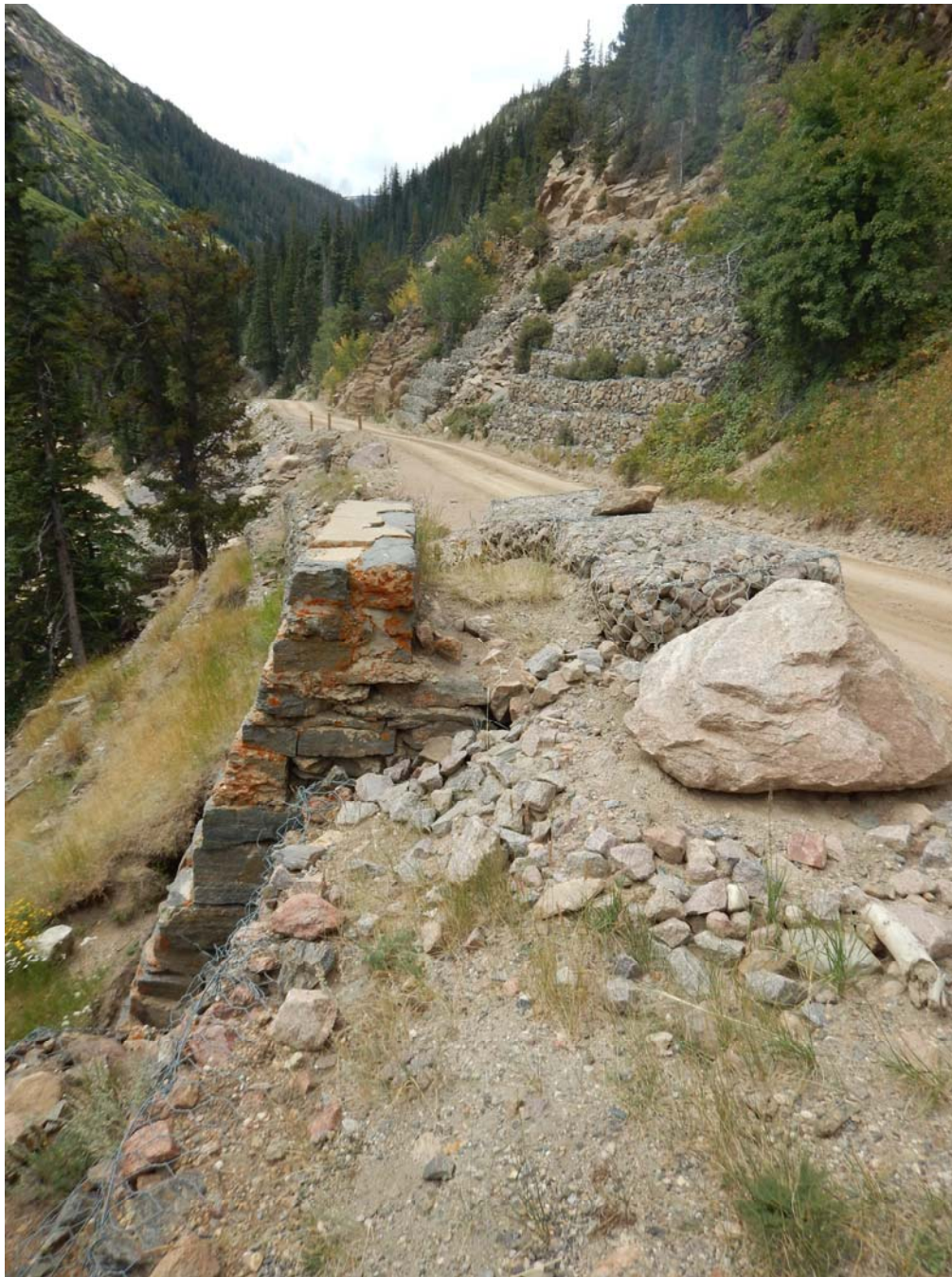
Photograph 18. Gabion and retaining wall, camera facing west. CO_LarimerCounty_Fall River Road_Amendment_Boundary Increase_Rocky Mountain National Park MRA_0018
