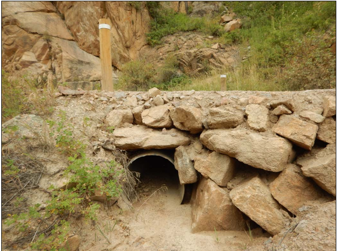
Photograph 1. Corrugated pipe culvert, camera facing northeast. CO_LarimerCounty_Fall River Road_Amendment_Boundary Increase_Rocky Mountain National Park MRA_0001
