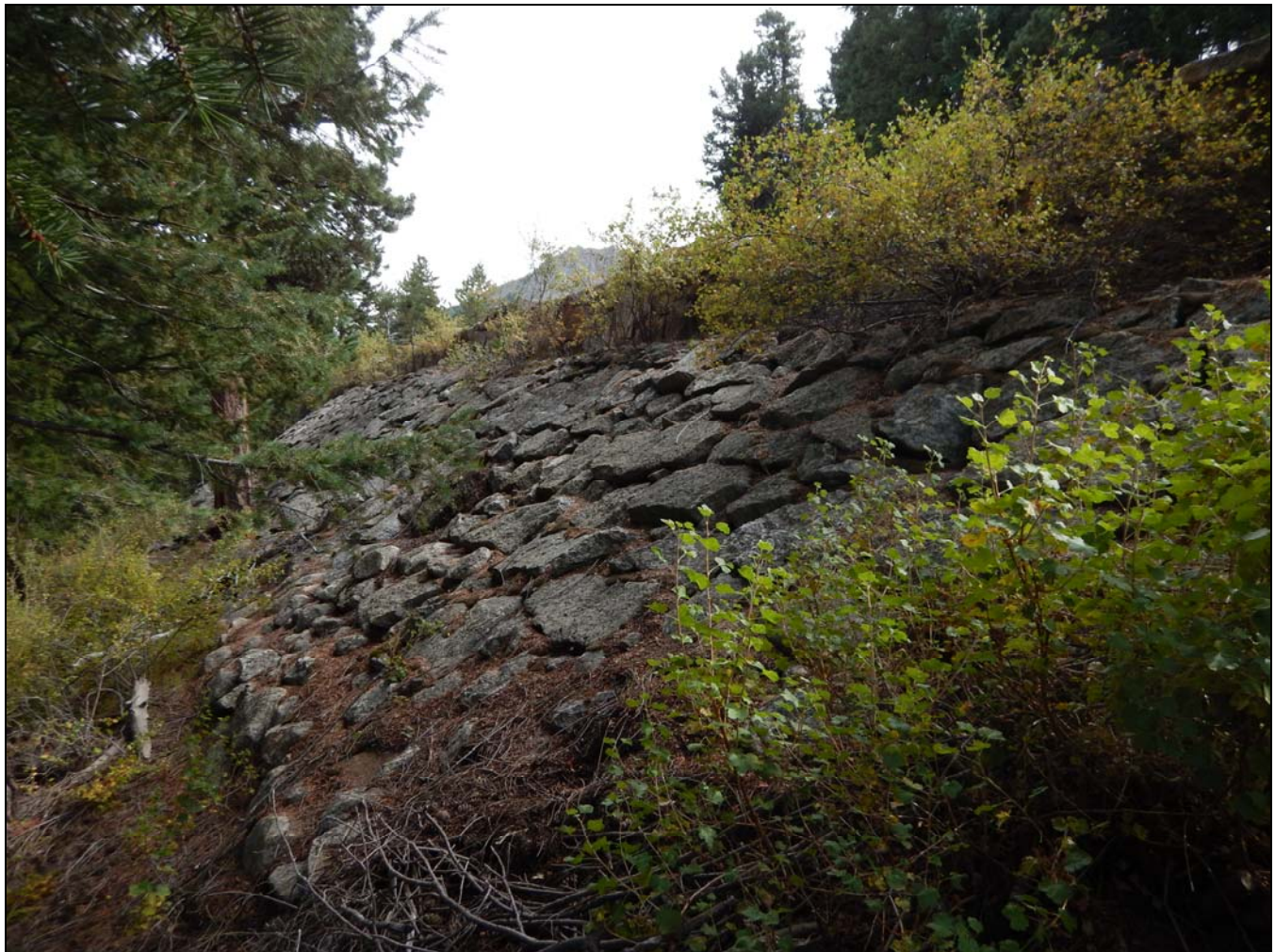
Photograph 7. Guard wall revetment, camera facing southwest. CO_LarimerCounty_Fall River Road_Amendment_Boundary Increase_Rocky Mountain National Park MRA_0007
