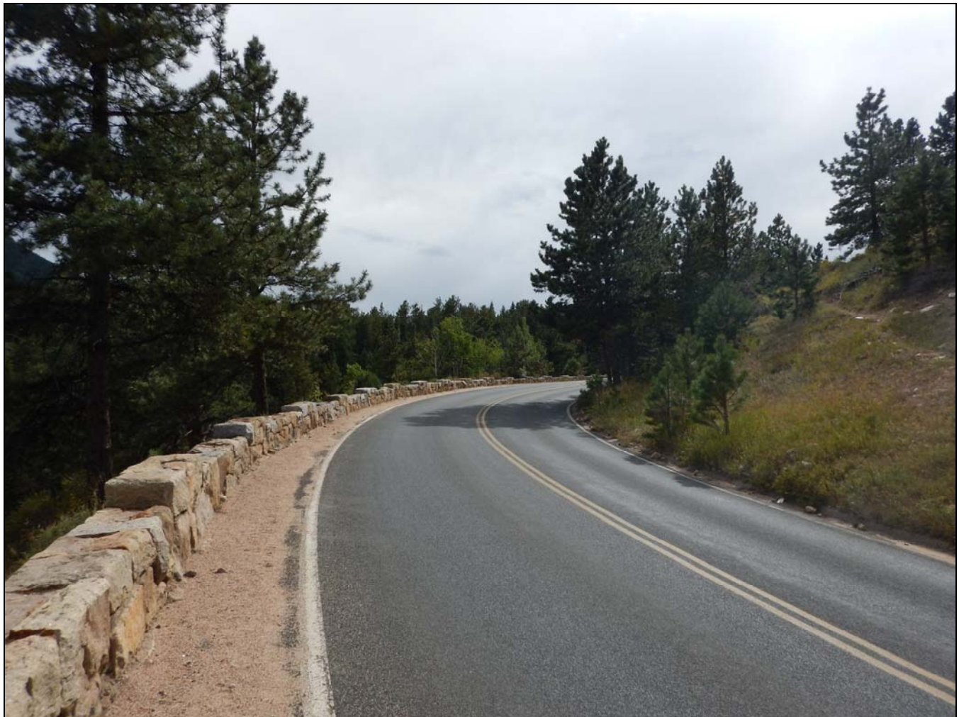
Photograph 6. Guard wall, camera facing south. CO_LarimerCounty_Fall River Road_Amendment_Boundary Increase_Rocky Mountain National Park MRA_0006
