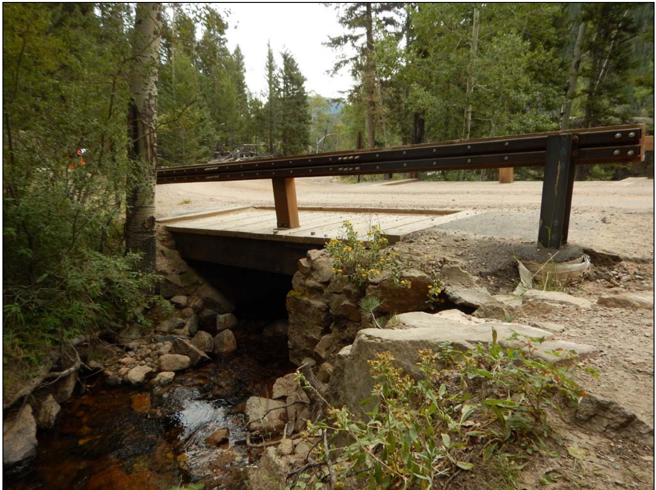
Photograph 11. Roaring River Bridge, camera facing southeast. CO_LarimerCounty_Fall River Road_Amendment_Boundary Increase_Rocky Mountain National Park MRA_0011
