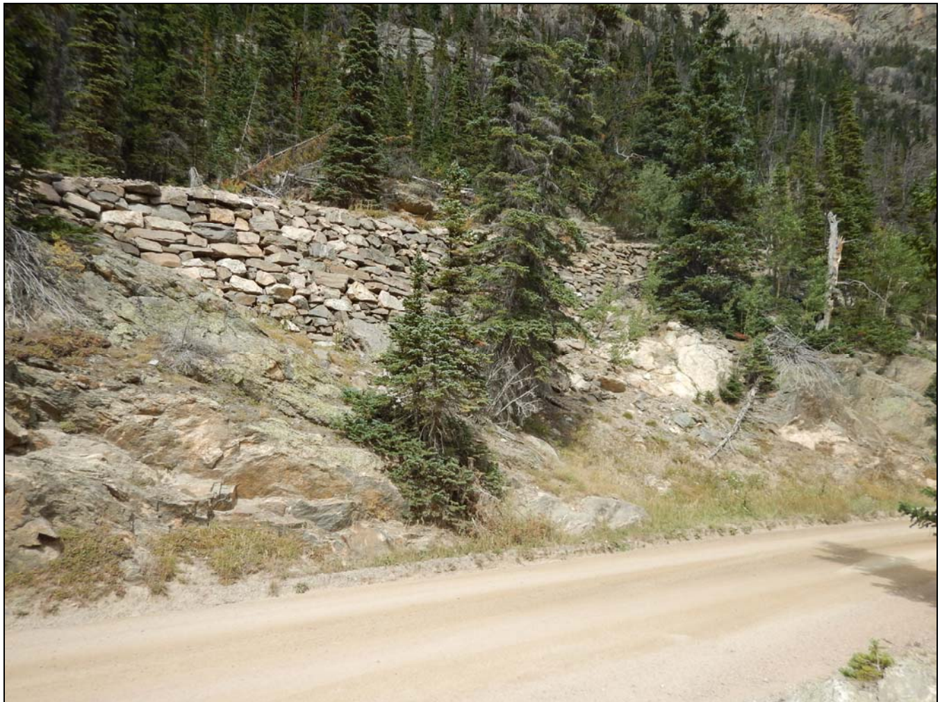
Photograph 8. Retaining wall, camera facing southeast. CO_LarimerCounty_Fall River Road_Amendment_Boundary Increase_Rocky Mountain National Park MRA_0008
