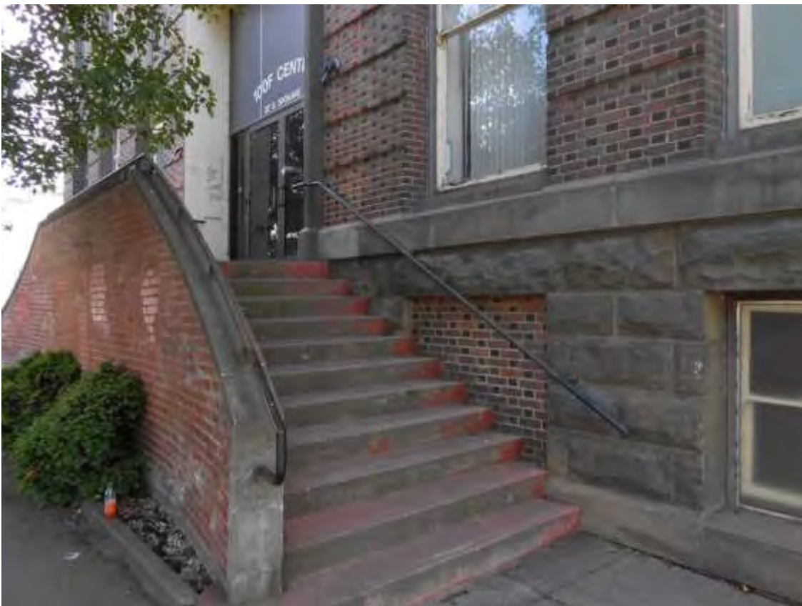
Fig. 5. Walla Walla, WA YMCA. Entry stair at 28 S. Spokane St., original 1907 masonry with 1948 alterations to entry stair, looking SW, June 2014. Source: Stephen Day Architecture.
