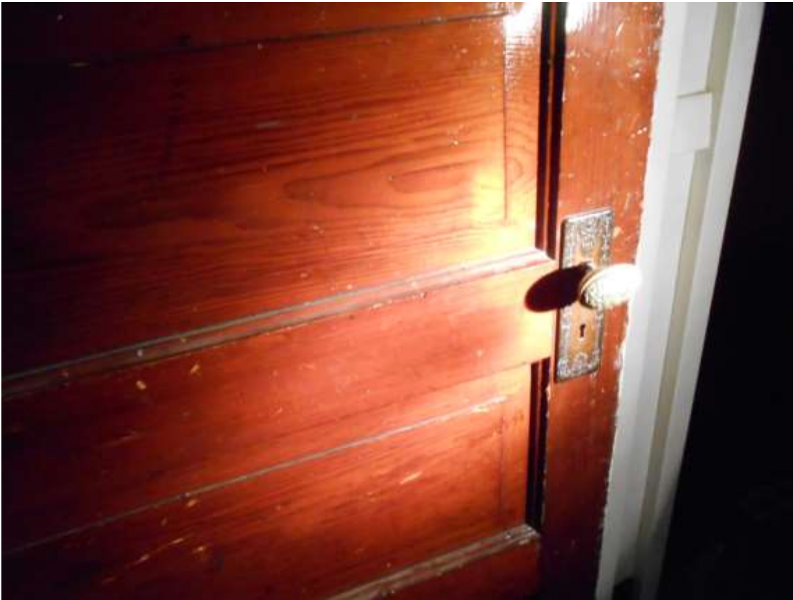
Fig.18. Walla Walla, WA YMCA. Detail of 1907 stained and varnished door, with original hardware, First Floor, June 2014. Source: Stephen Day Architecture.
