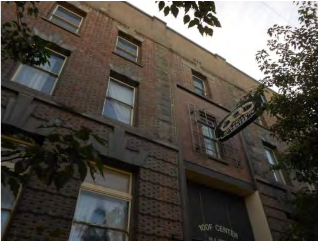
Fig. 6. Walla Walla, WA YMCA. East elevation detail, original masonry with 1948 window modifications at center bay, looking NW, June 2014. Source: Stephen Day Architecture.
