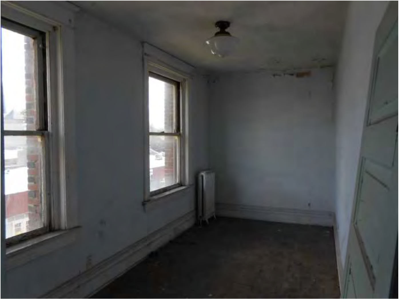
Fig. 27. Walla Walla, WA YMCA. Third floor lodging room, SE corner, window and base trim, possibly original light fixture, radiator, view looking south, June 2014. Source: Stephen Day Architecture.
