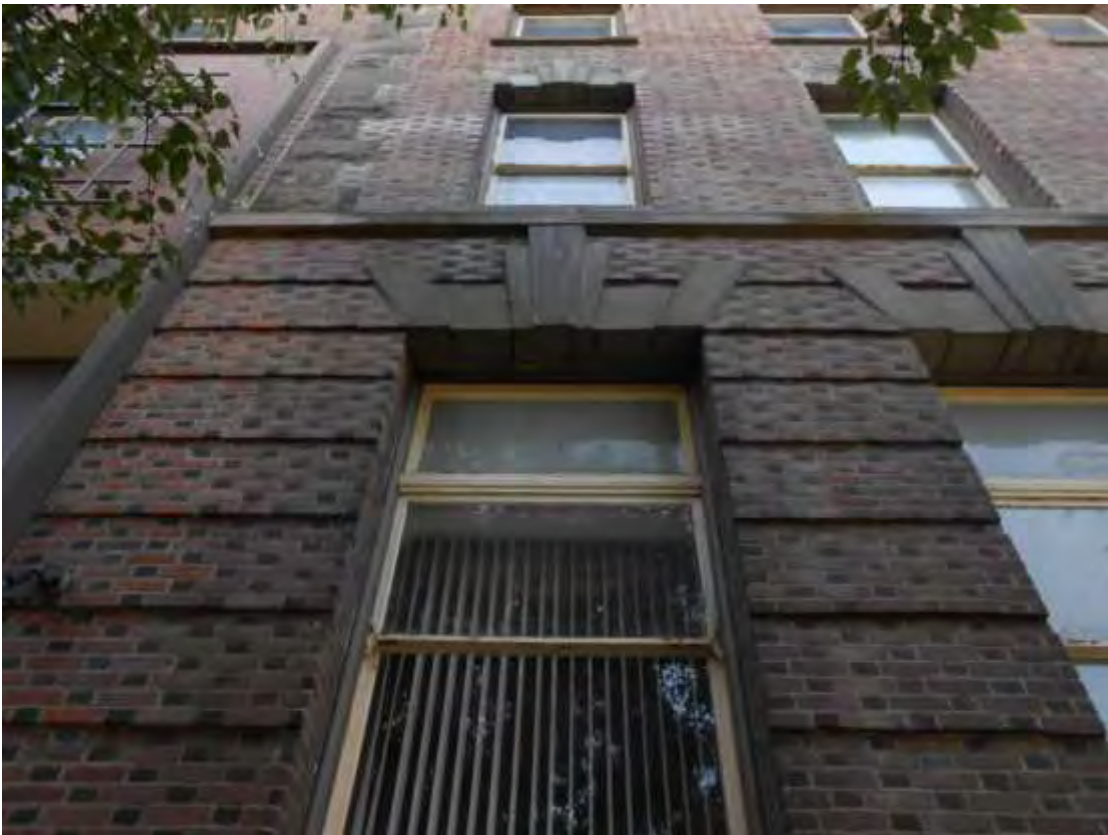
Fig. 3B. Walla Walla, WA YMCA. Detail of brick and sandstone masonry, original wood windows, east elevation, looking west, June 2014. Source: Stephen Day Architecture.
