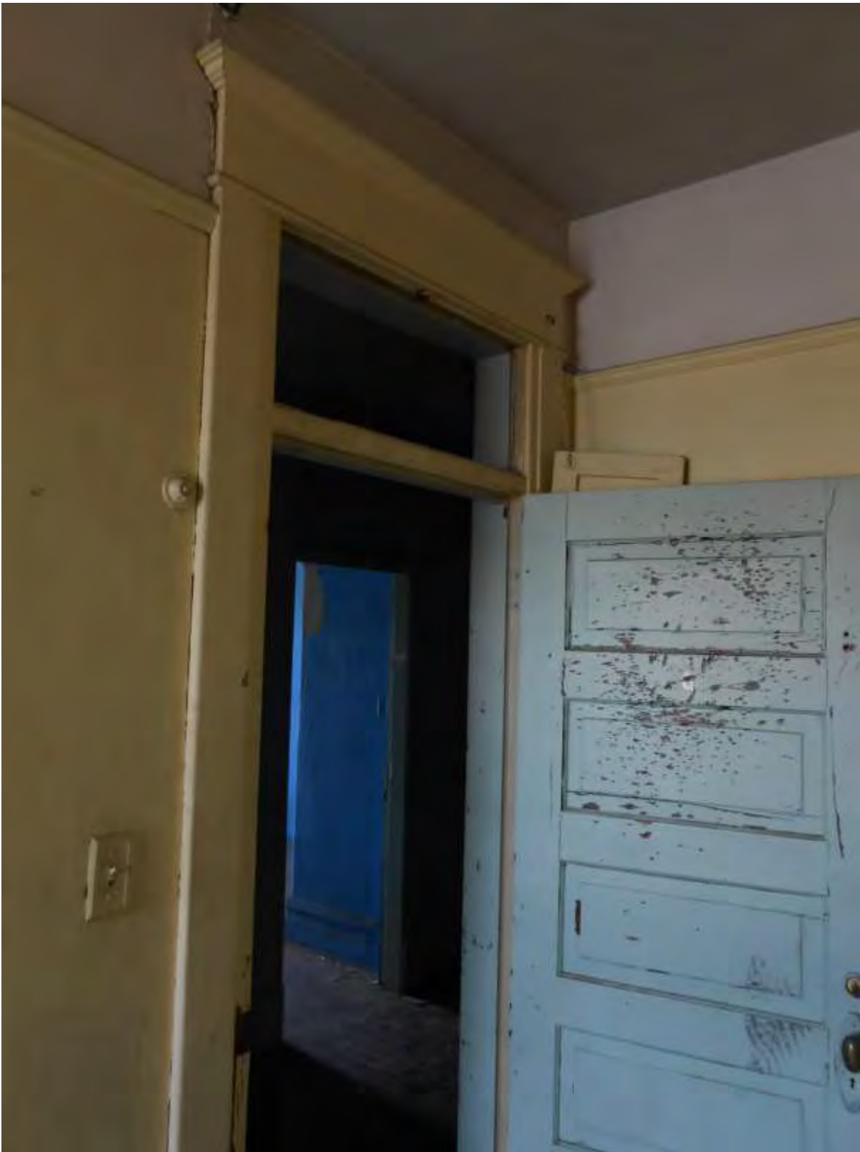
Fig. 26. Walla Walla, WA YMCA. Third floor lodging room door, casing, transoms, view looking east, June 2014. Source: Stephen Day Architecture.
