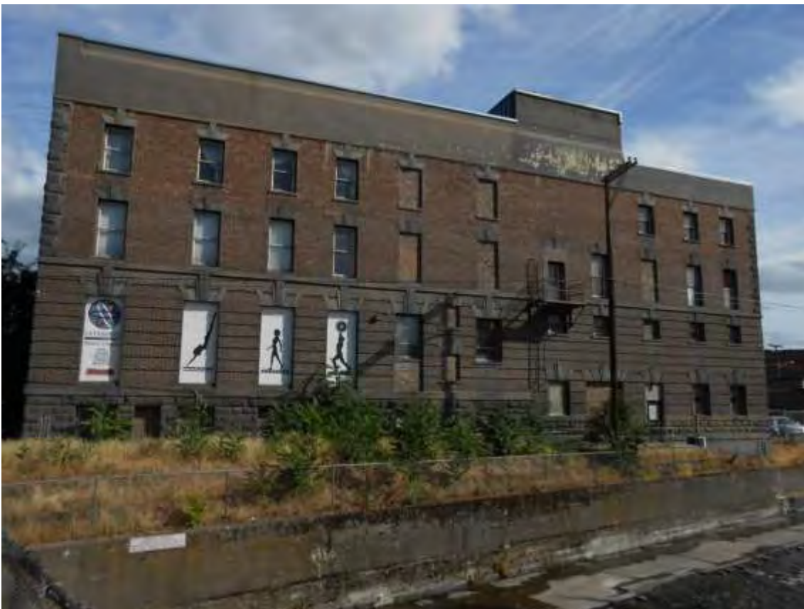
Fig. 9. Walla Walla, WA YMCA. North elevation facing Mill Creek waterway, looking south, June 2014. Source: Stephen Day Architecture.
