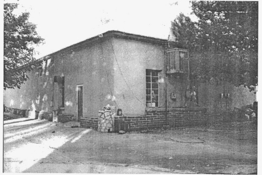
The rear of the building shows some of the minor alterations: the adobe-veneer water table, the plaster on the original adobe walls, and the steel casement windows.
