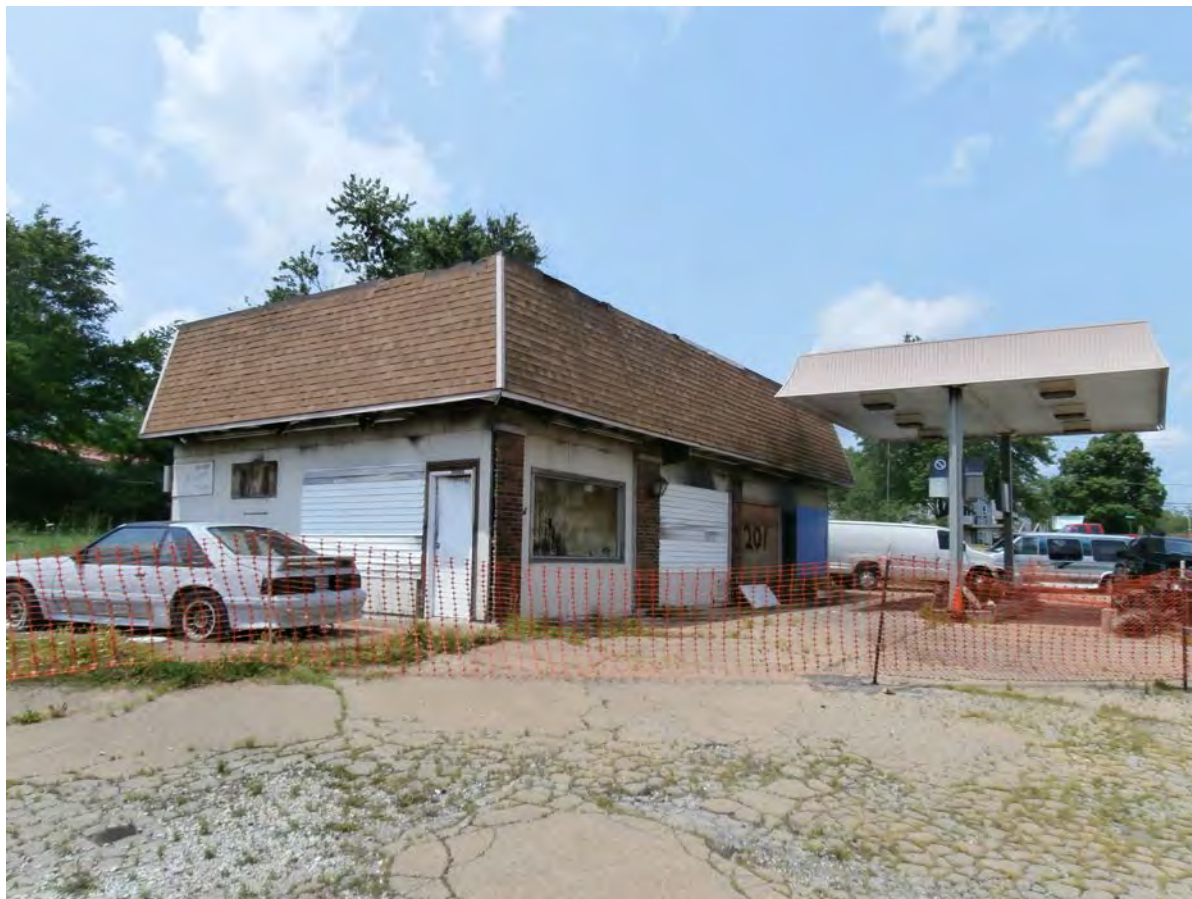
Figure 18. 201 S Front Street within the former city boundaries of Elvins appears out of use and recently suffered fire damage. Photographed by Amber Cox, June 1, 2019.
