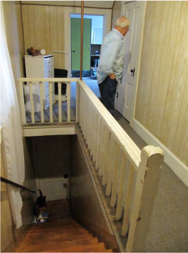
12 of 22: Stair balustrade and hallway on second floor, looking north in 2014 prior to rehab
