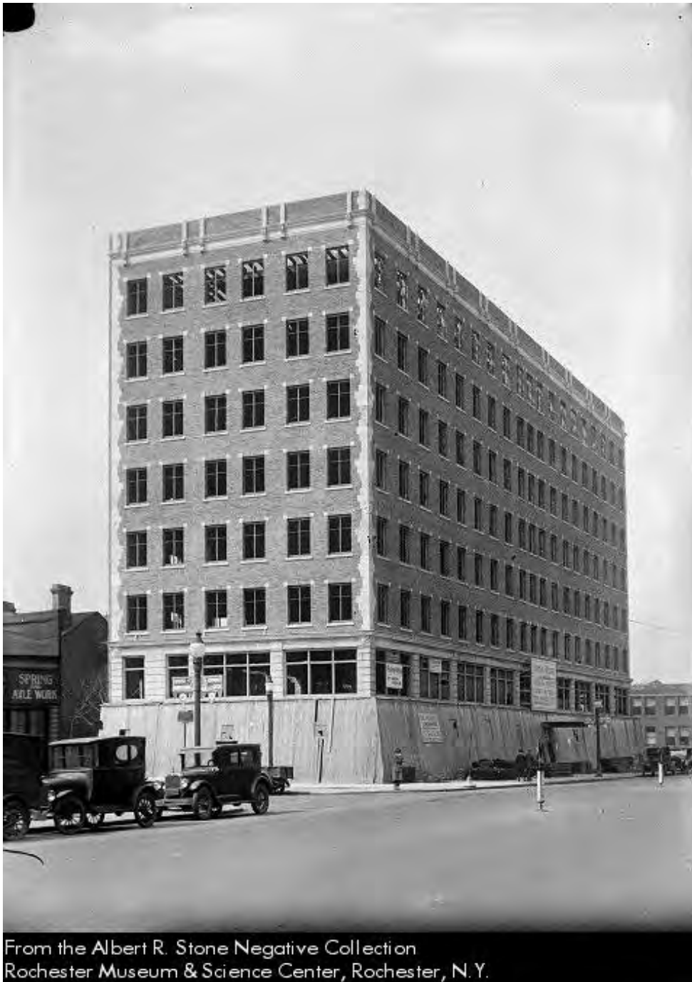
The Terminal Building under construction, c.1925-1926. Albert R. Stone Negative Collection. Rochester Museum & Science Center.
