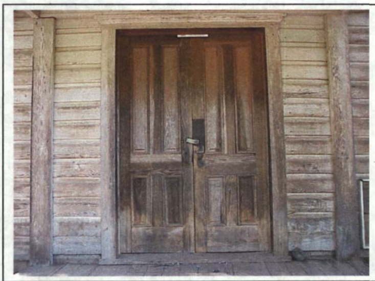
Plate 6. Detail of doors with scale.
