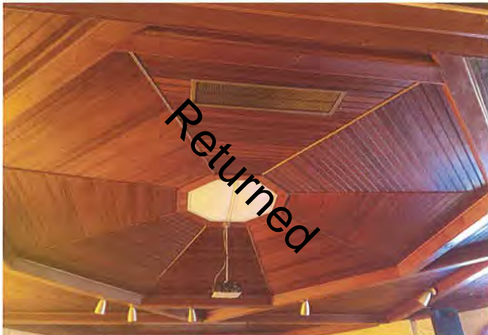
Image 3: The ceiling is oak, laid in an octagonal pattern that corresponds with the ceiling framing that allows the clear-span over the main sanctuary. (The ceiling is below a standard pyramidal roof, the actual roof structure is not an octagonal form.)
