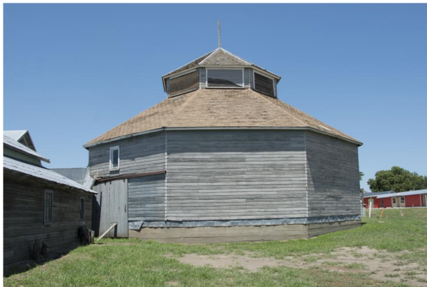
Photo #2 (NE_Red Willow County_Bartley Sales Barn_0002) Close-up of south façade, camera facing north.
