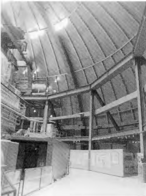
Steel rail frame
