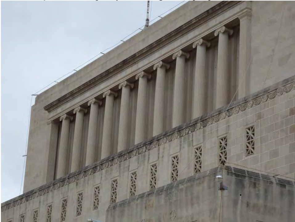
Photo 4: Façade, detail of peristyle and swag around parapet of second tier, March 30, 2016, looking southwest.
