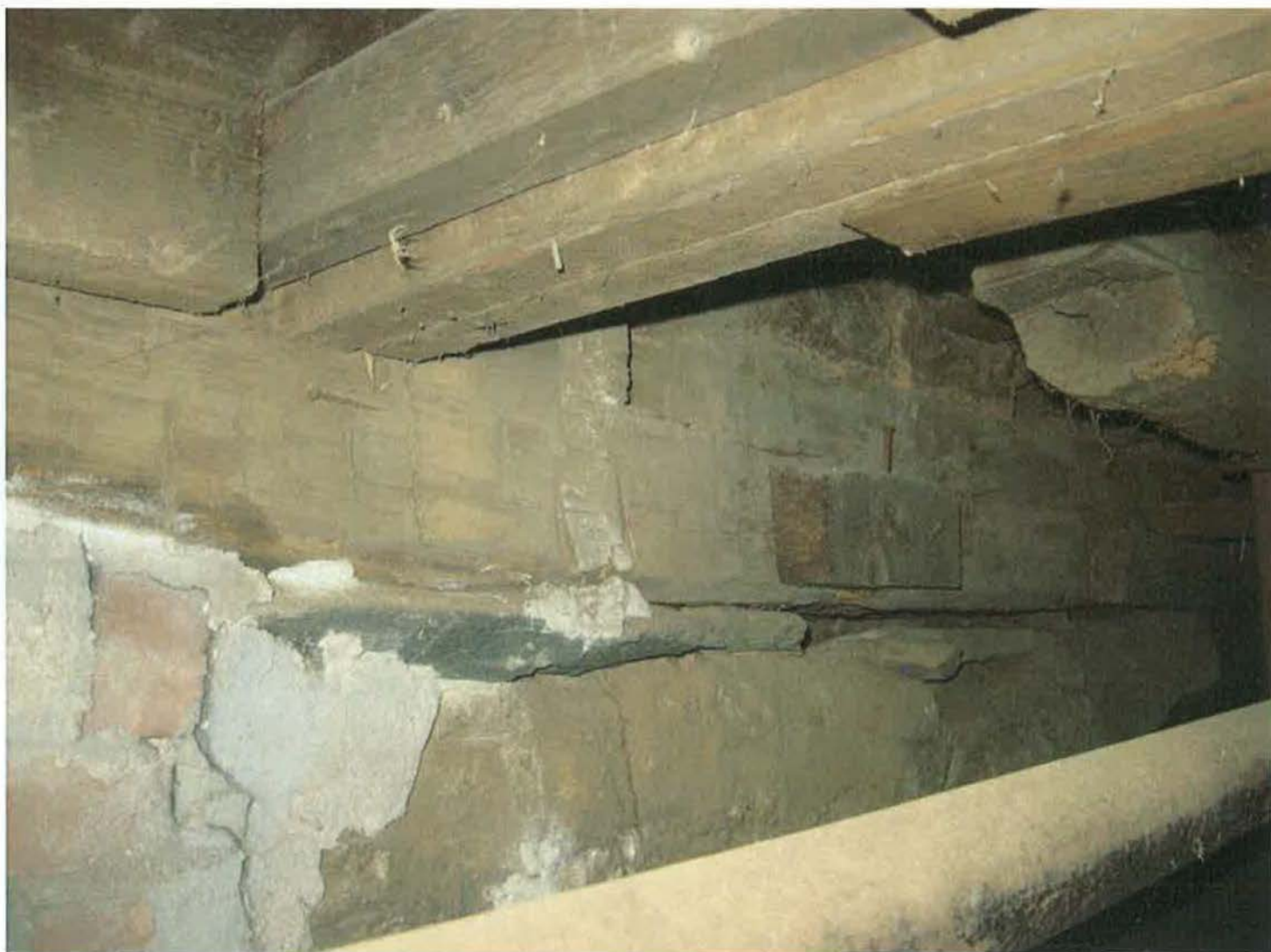
Interior of cellar, showing original chimney girt and early-twentieth-century floor joist details. Camera facing northeast. Photograph 12 of 27.
