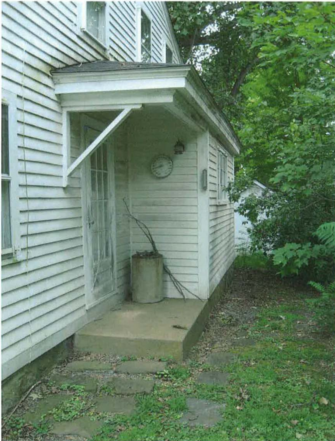
North (side) elevation, showing rear ell and side entry porch. Camera facing west. Photograph 10 of 27.
