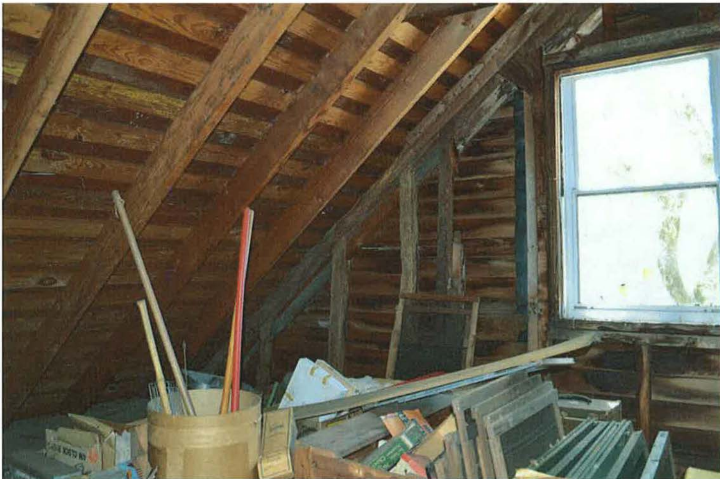
Interior of attic, showing wall, roof, and window details. Camera facing south. Photograph 24 of 27.
