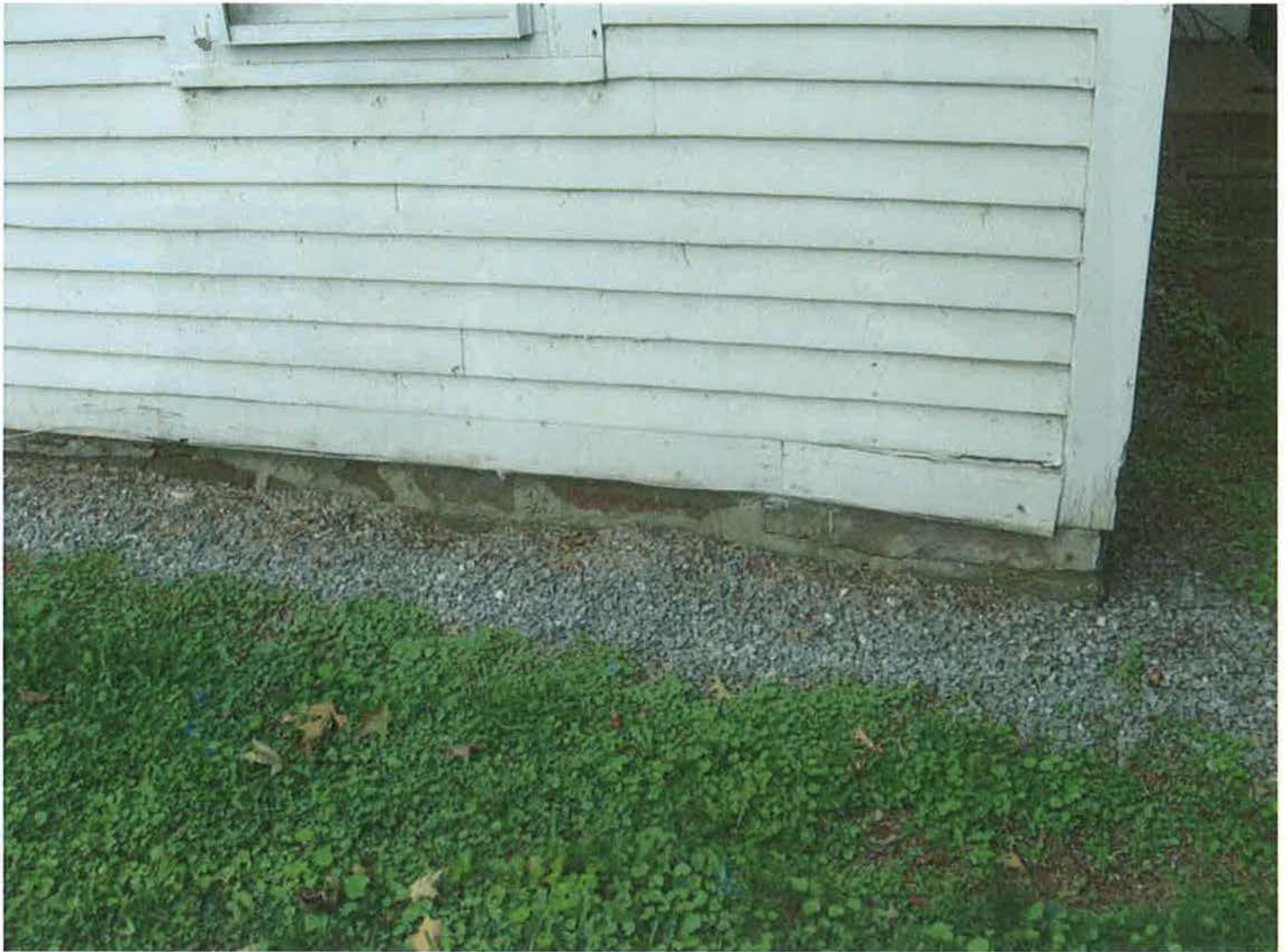
East (front) and north (side) elevations of house from Main Street, showing foundation, corner board, and window trim details. Camera facing west. Photograph 4 of 27.
