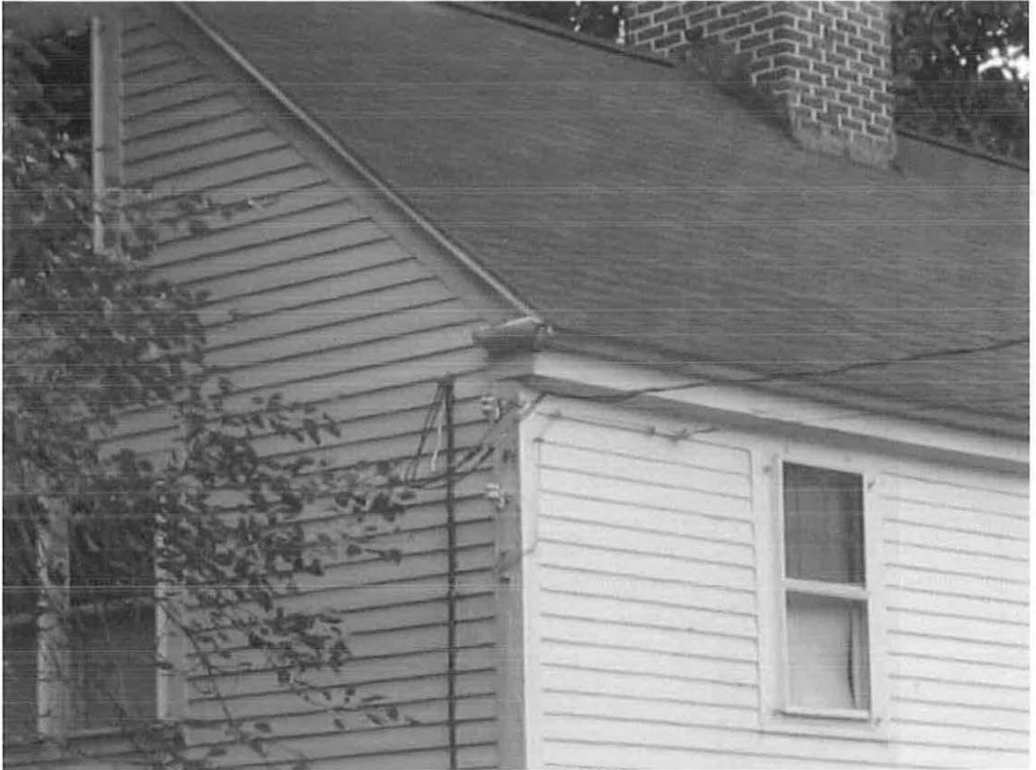
East (front) and south (side) elevations of house from Main Street, showing cornice and rakeboard details.
