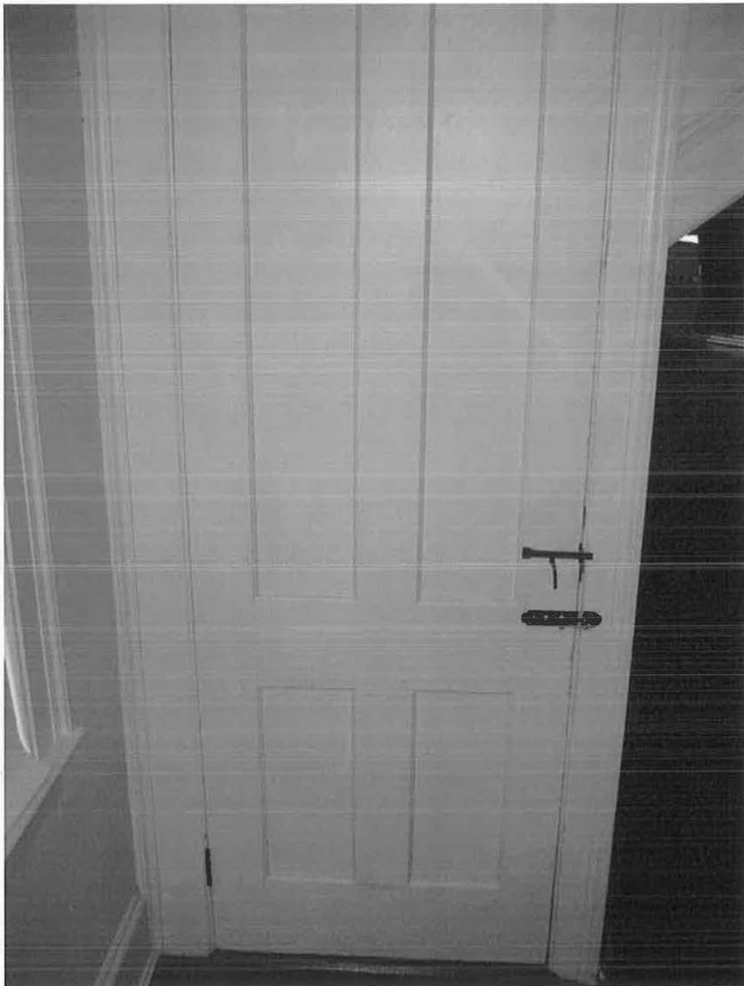
Interior of hall, showing cellar access door details. Camera facing west. Photograph 11 of 27.
