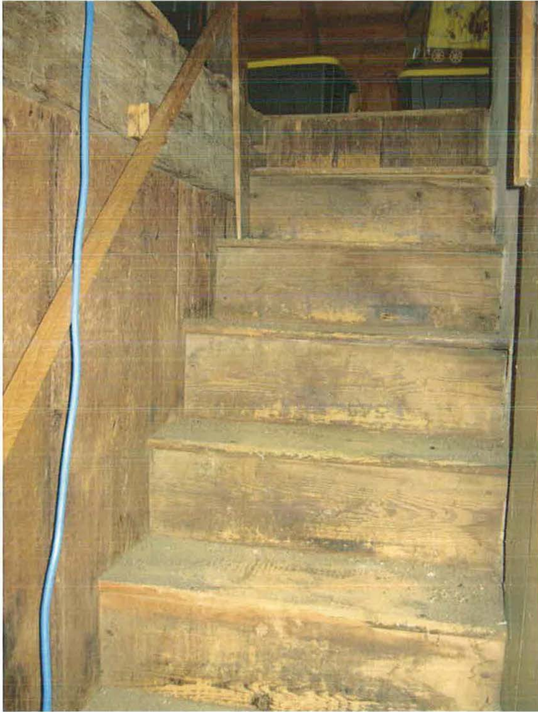
Interior of attic stairwell, showing stair and wall details. Camera facing east. Photograph 23 of 27.
