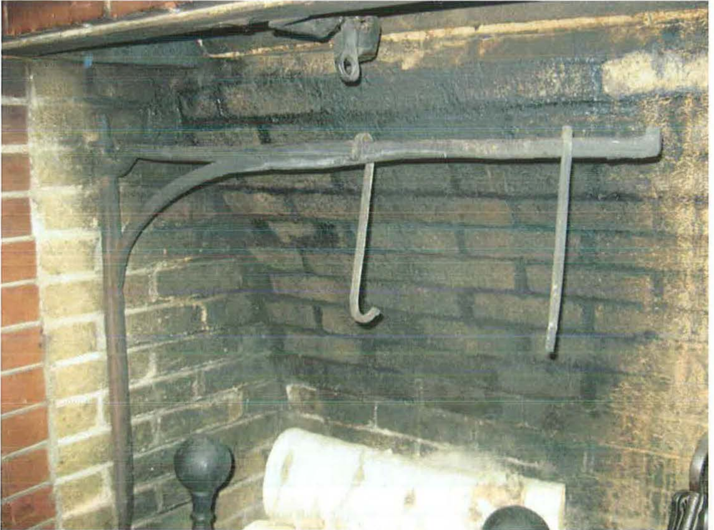
Interior of original kitchen, first floor of house, showing fireplace details. Camera facing east. Photograph 21 of 27.
