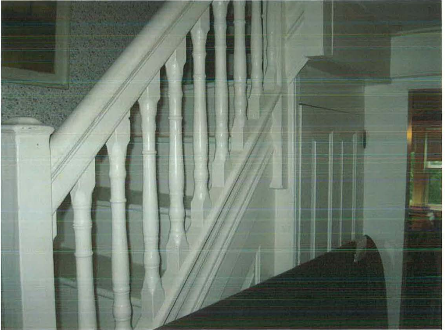
Interior of entry hall, showing stair, newel post, rail, baluster, paneling, and door details. Camera facing north. Photograph 13 of 27.
