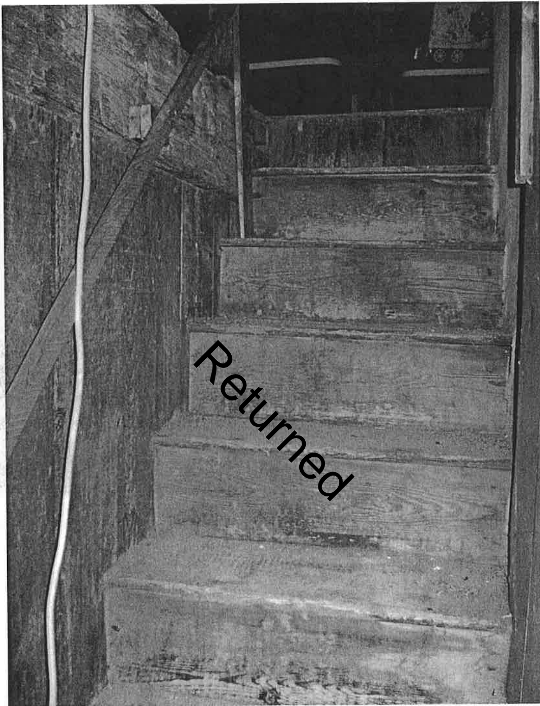
Interior of attic stairwell, showing stair and wall details. Camera facing east. Photograph 23 of 27.
