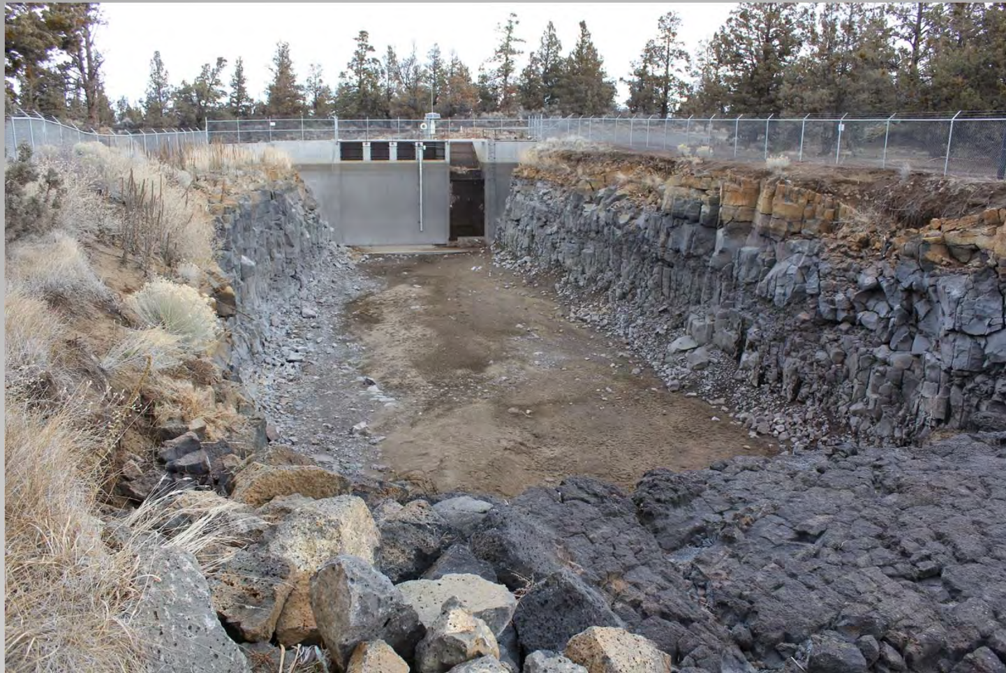
Just north of the Historic District is the intake to the Juniper Ridge Hydroelectric Project 9-foot diameter pipe.
