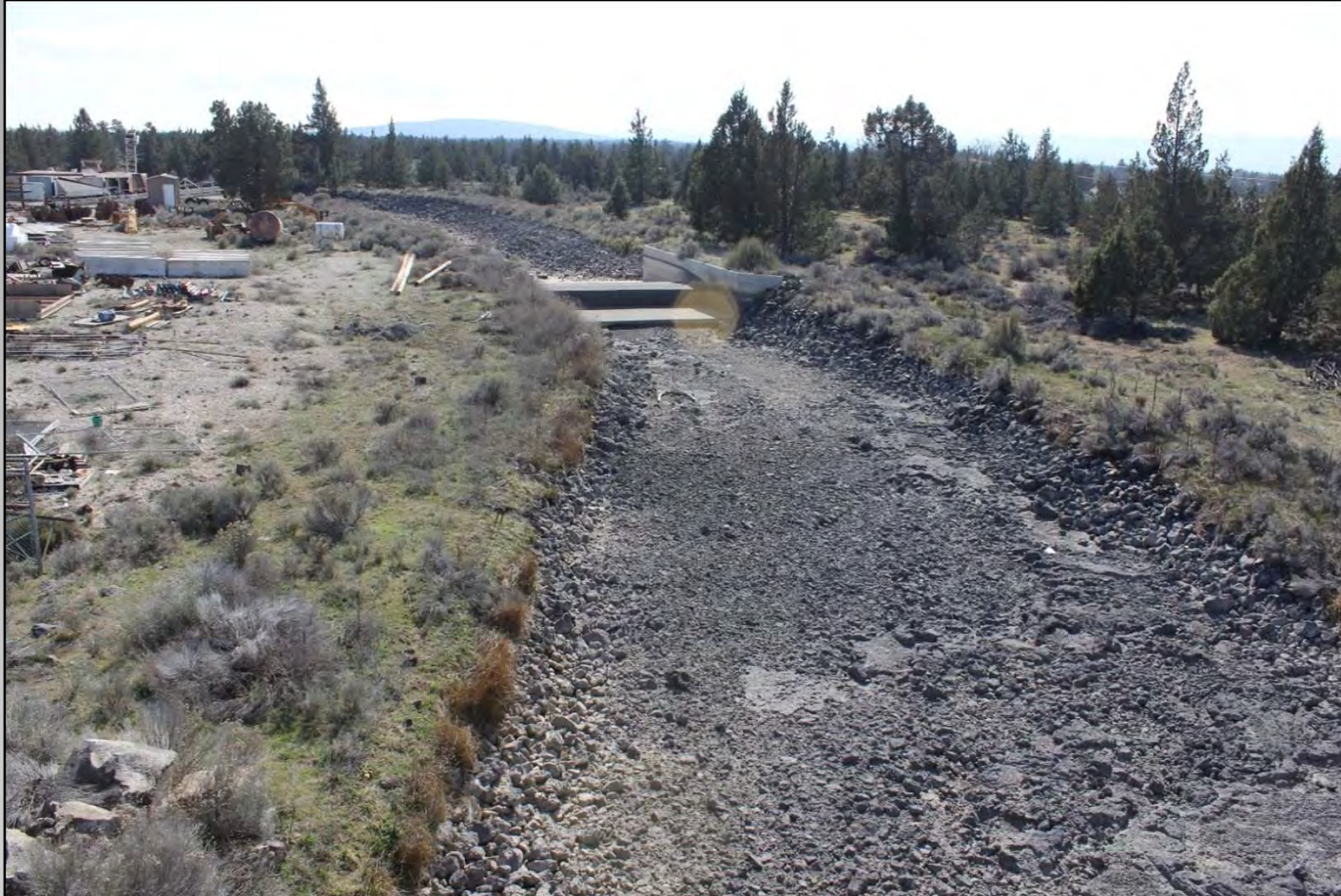
Flow Measuring Weir at Deschutes Junction
