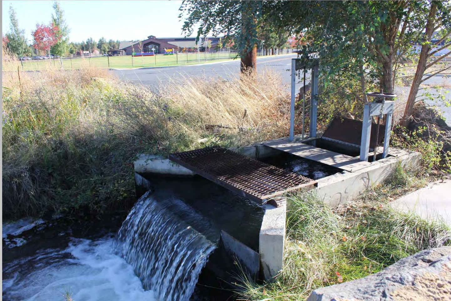
The A-4 Lateral comes out of pipe at gate at Old Deschutes Road near Ponderosa Elementary School, and heads northeast.
