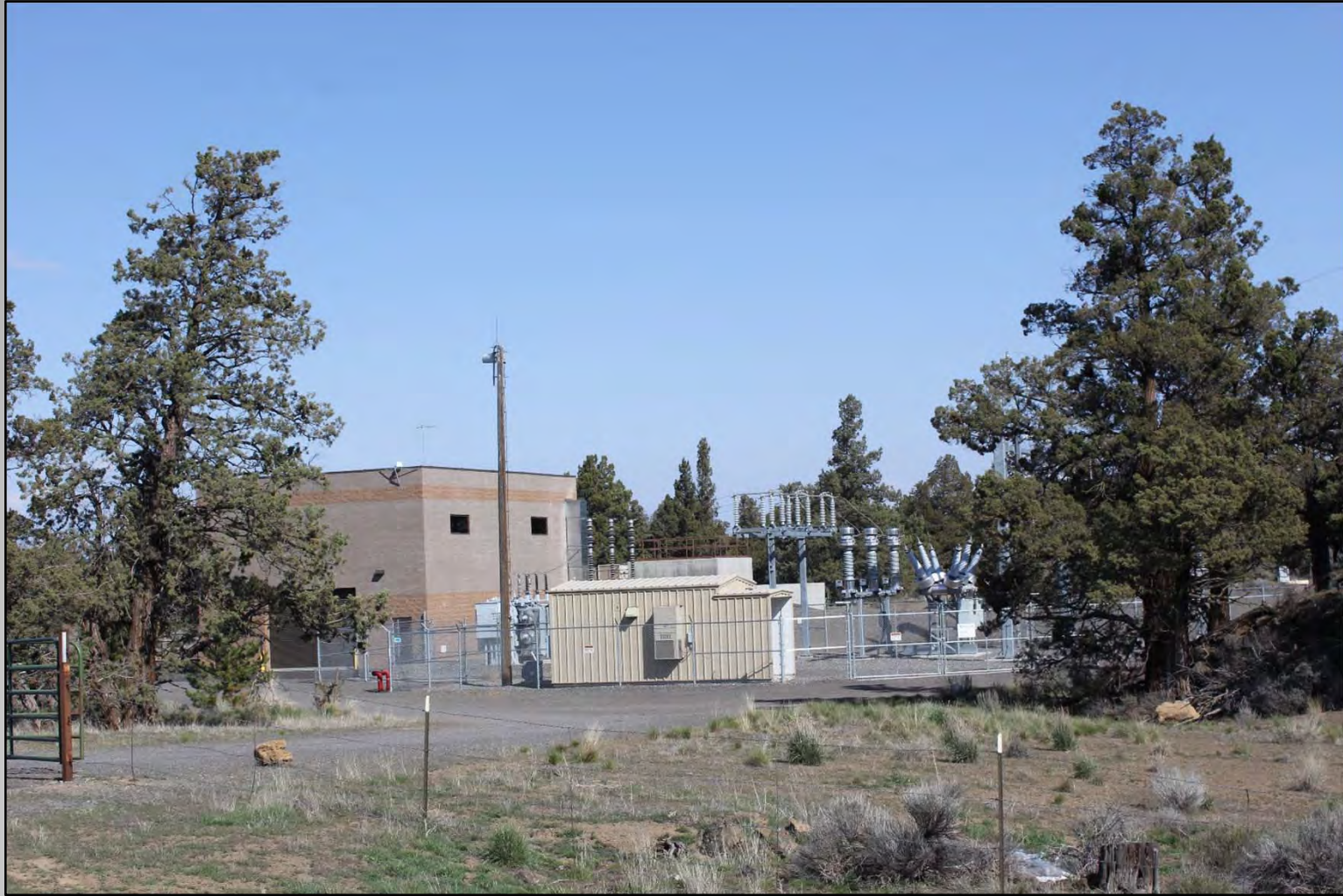
Juniper Ridge Hydroelectric Plant
