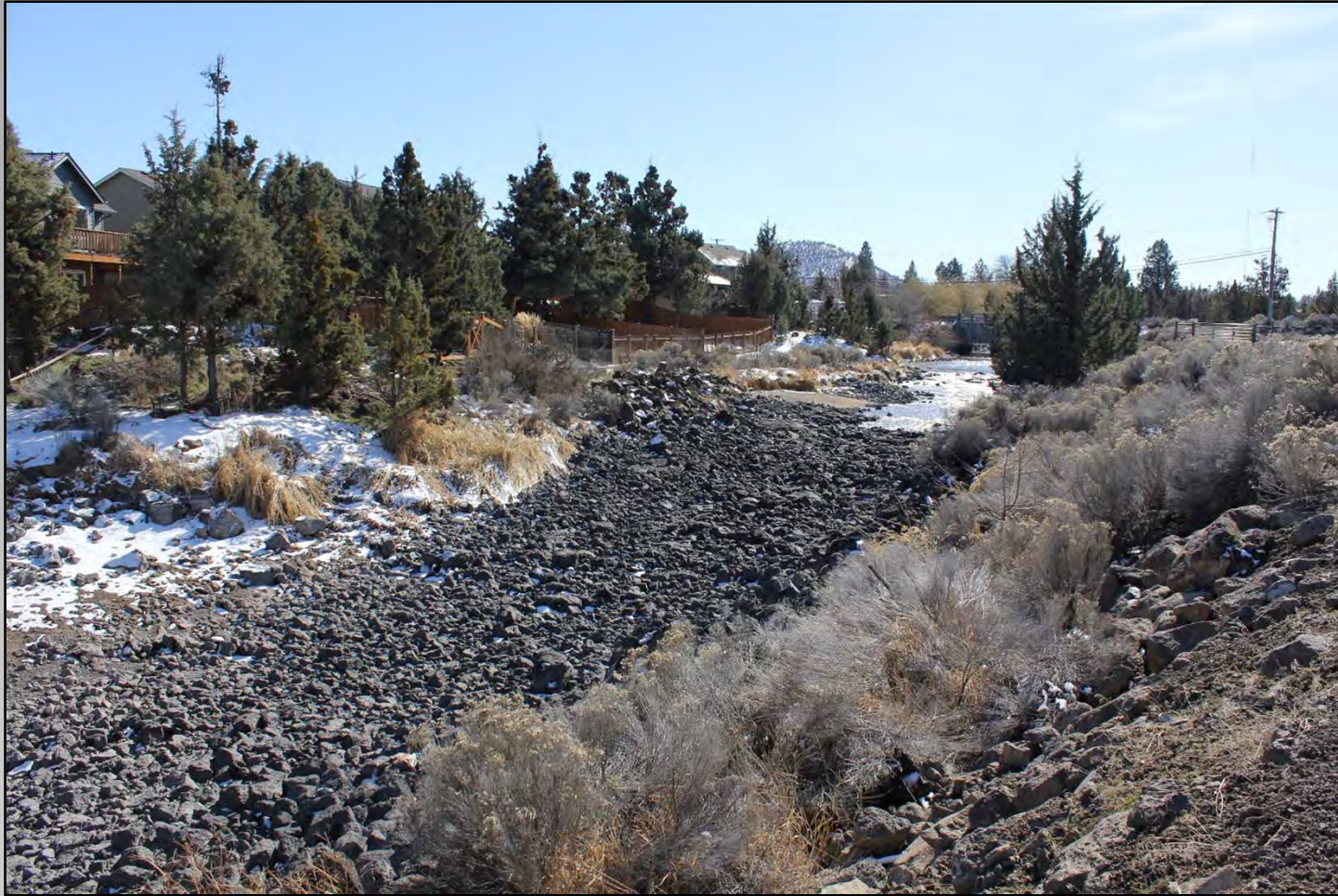
Looking south toward Pilot Butte. Houses on left. Loose rock in bed of undulating Pilot Butte Canal. Crude construction.
